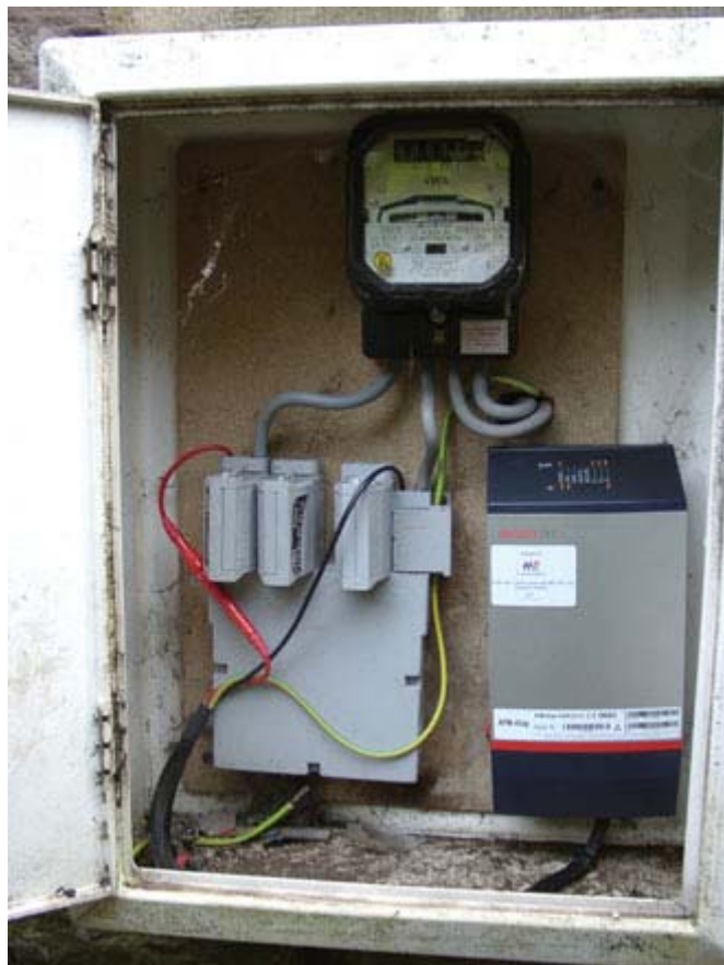
Fig. 2. The Ascom Outdoor Access Point, installed in an outdoor meter cupboard. The OAP is the unit in the lower right of the picture, and, as can be seen, was connected to the supply side of the electricity meter. (At the other Ascom-equipped premises visited there was an electrically similar arrangement, but in that case the meter and OAP were housed indoors.)
